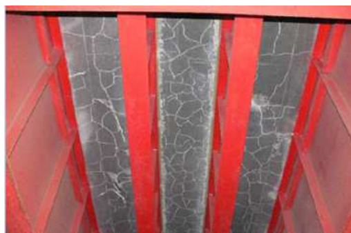
(C) 橋梁床版のひび割れ
